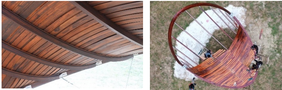
Figure 13. a) Sealing of gap between catenary beam and roof planks, b) Discretising the area of highest curvature.
