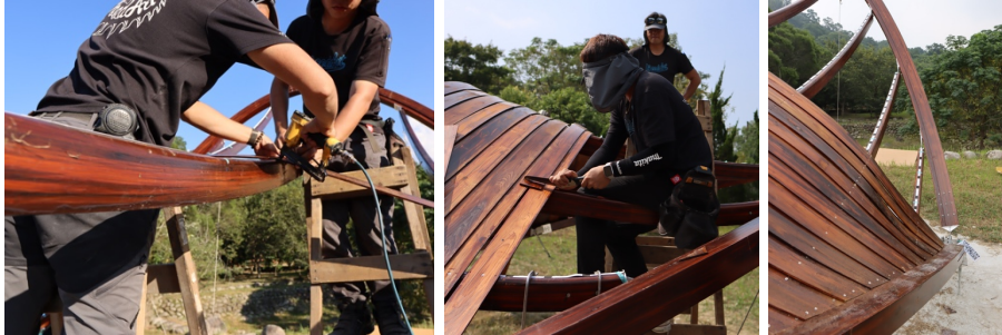
Figure 11 a) Wooden plank nailing, b) In-situ plank trimming, c) Reference guides for plank pattern
